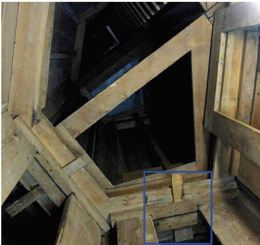
8. A wedge mortise and tenon joint (blue colour) on a frame of a module inside the altarpiece. Photo: Disent AB.
